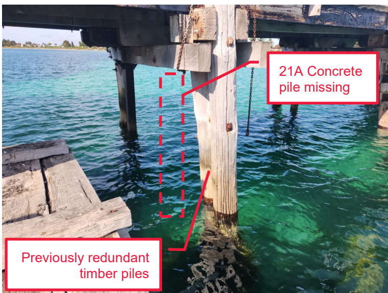
Figure 6: Bent 21A Pile Missing and Redundant Timber Pile
