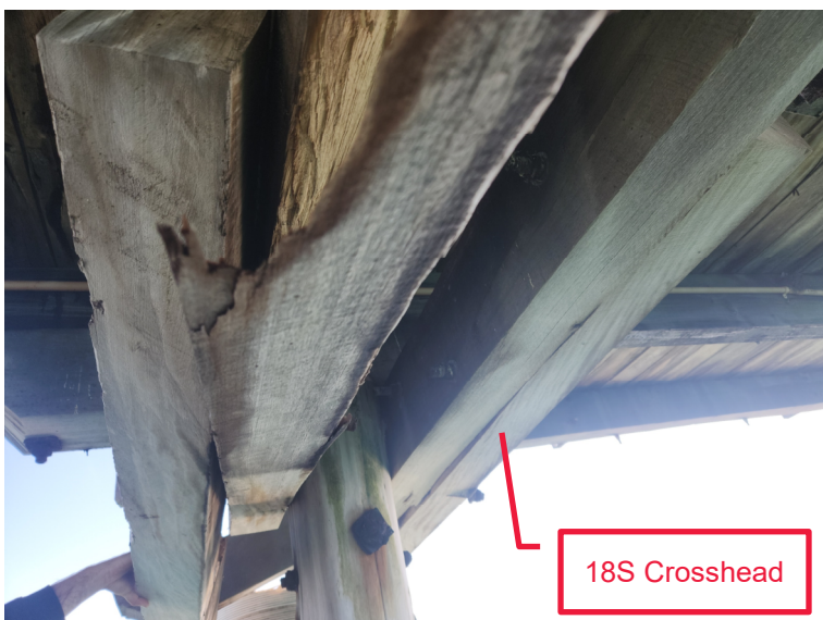
Figure 3: Bent 18S Crosshead Splitting
