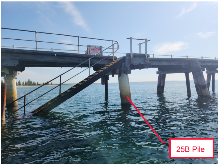
Figure 8: Bent 25B Pile Failure and Rotation
