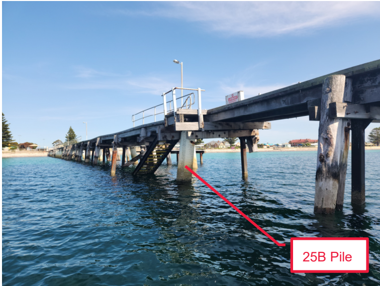
Figure 7: Bent 25B Pile Failure
