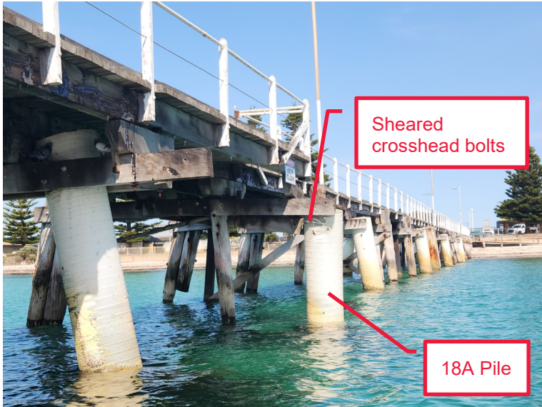
Figure 4: Bent 18A Pile Failure and Dropping
