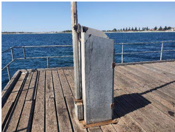
Figure 35 – Typical Condition 4 Navigation Beacon (Defect: Surface Corrosion)
