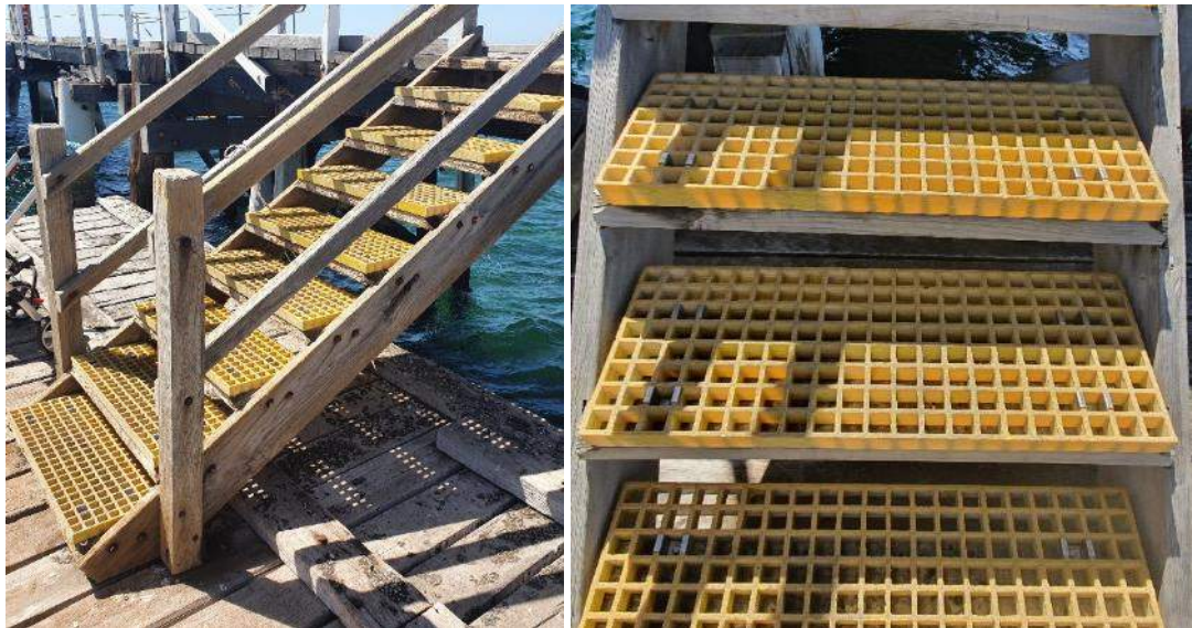
Figure 41 – Typical Landing Stair Defects (Defect: Weathering)
