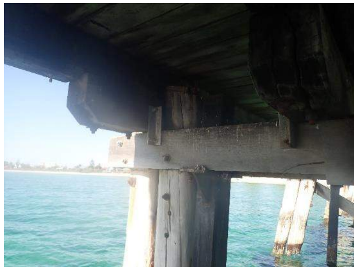
Figure 16 – Typical Condition 4 Timber Crosshead (Defect: Weathering)
