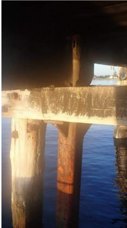
Figure 11 – Typical Condition 5 Steel Pile (Defect: Surface Corrosion & Pitting)
