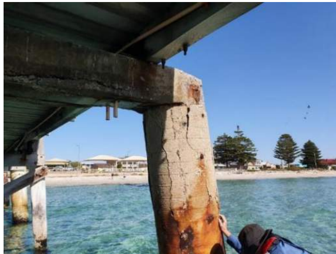
Figure 14 – Typical Condition 6 Concrete Pile (Defect: Missing sleeve, cracking and spalled concrete along pile)
