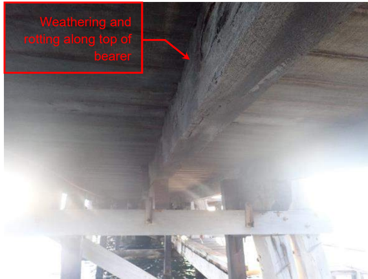
Figure 24 – Typical Condition 5 Bearer (Defect: Splitting and Weathering along Top)
