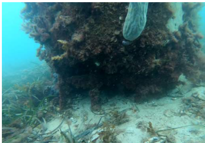
Figure 15 – Typical Condition 7 Concrete Pile (Defect: Missing sleeve, exposed reinforcement and missing concrete at seabed)
