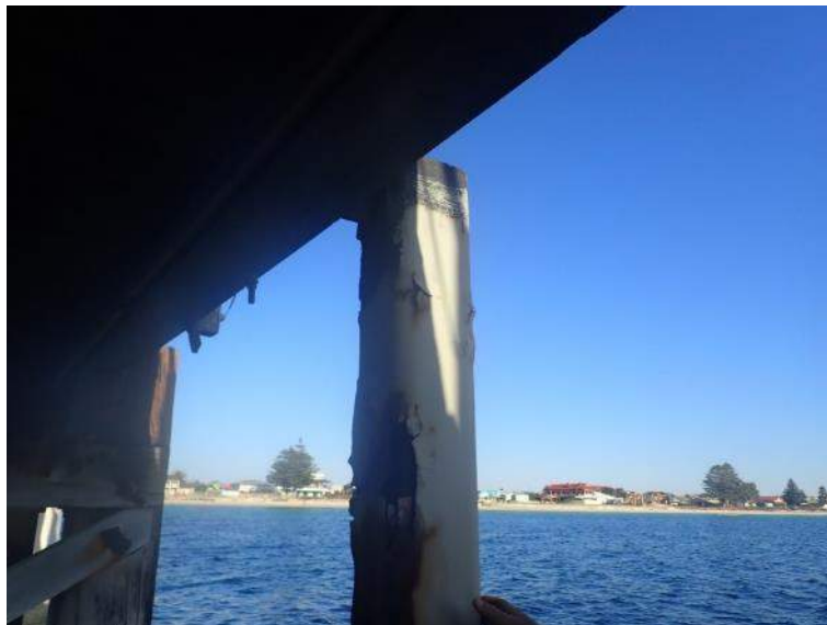
Figure 12 – Typical Condition 6 Steel Pile (Defect: Surface Corrosion, Pitting & Section Loss)
