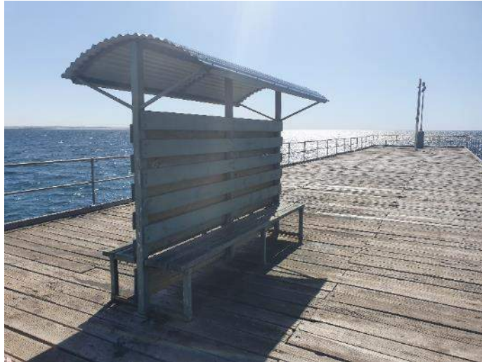
Figure 33 – Typical Condition 4 Shelter (Defect: Surface Corrosion & Weathering)
