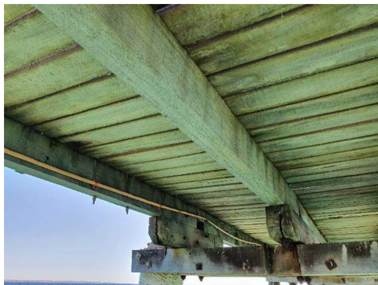
Figure 23 – Typical Condition 3 & 4 Bearer (Defect: Minor Splitting & Weathering)
