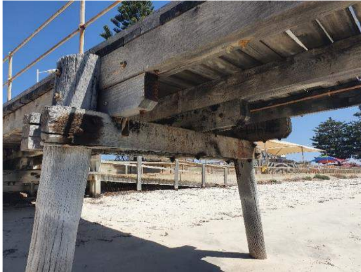
Figure 17 – Typical Condition 5 Timber Crosshead (Defect: Splitting at Ends and Weathering)
