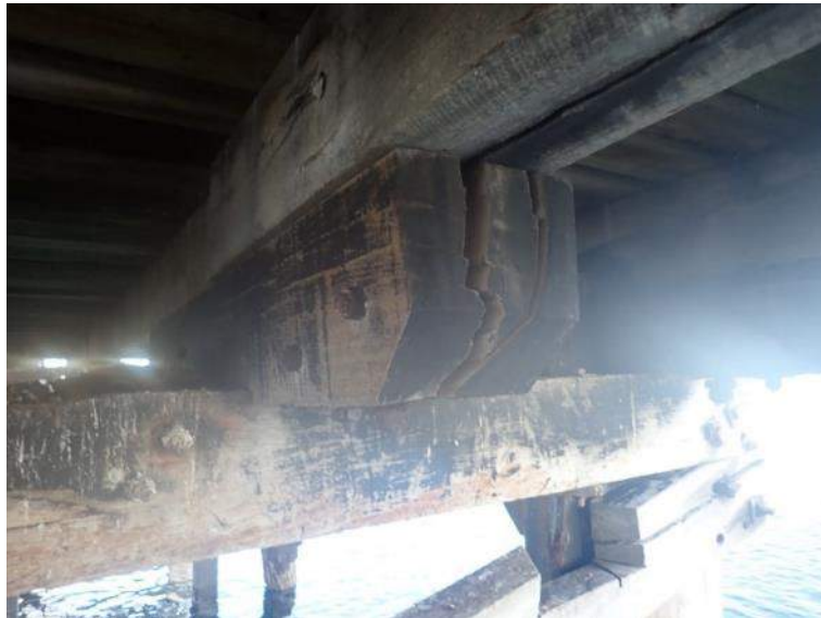
Figure 22 – Typical Condition 6 Timber Corbel (Defect: Weathering & Major Splitting Along Member)
