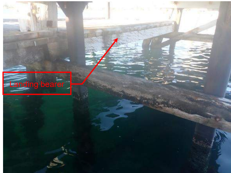
Figure 38 – Typical Condition 4 & 5 Landing Bearer, In Rear Ground (Defect: Splitting & Weathering)
