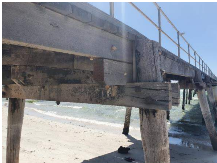
Figure 20 – Typical Condition 3&4 Timber Corbel (Defect: Weathering & Minor Splitting of Member)
