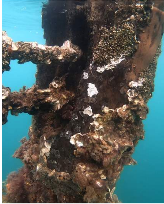
Figure 7 – Typical Condition 5 Timber Pile (Defect: Necking & Damage at cross brace)
