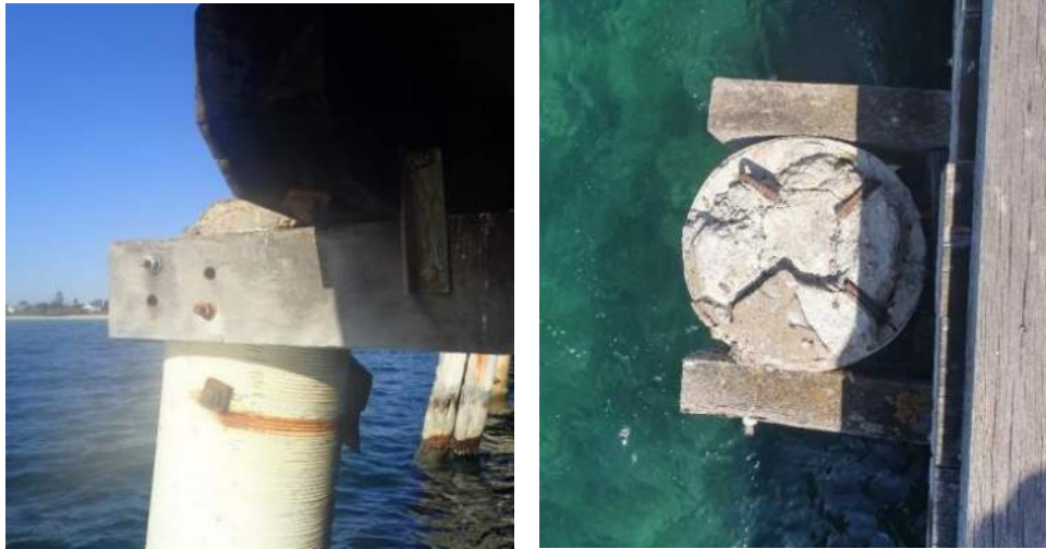
Figure 13 – Typical Condition 5 Concrete Pile (Defect: Minor damage to sleeve, exposed reinforcement and spalled concrete)
