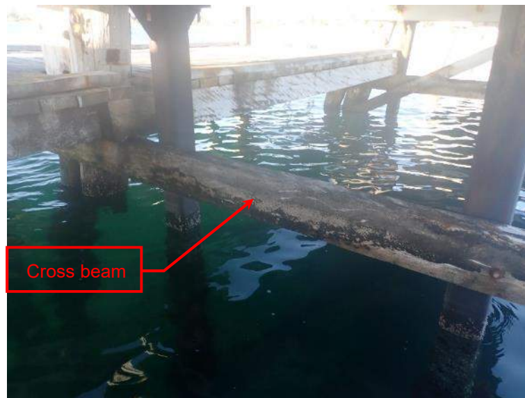
Figure 27 – Typical Condition 4/5 Crossbeam (Defect: Minor Splitting and Weathering)
