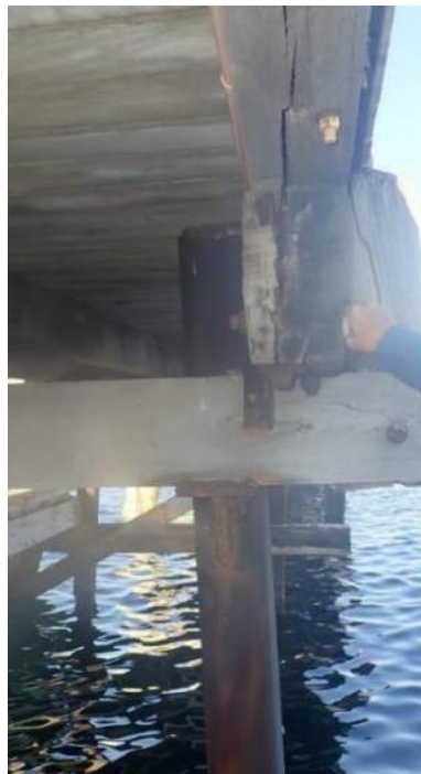
Figure 10 – Typical Condition 4 Steel Pile (Defect: Surface Corrosion)
