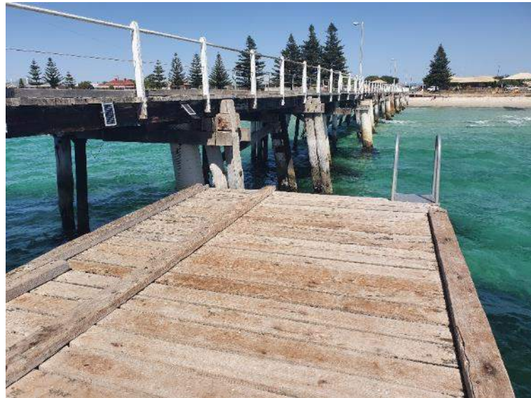
Figure 40 – Typical Condition 4 & 5 Timber Kerbing (Defect: Splitting & Weathering)
