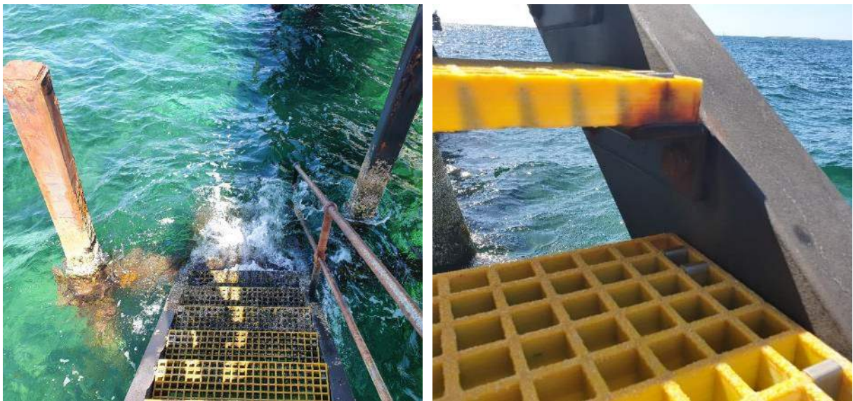
Figure 36 – Typical Access Stair Defects (Defect: Corrosion)
