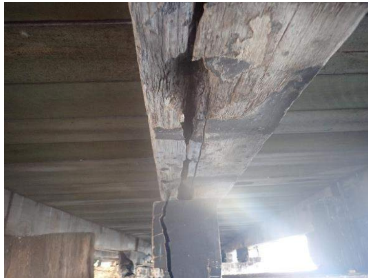
Figure 25 – Typical Condition 6 Bearer (Defect: Major Splitting & Rotting)
