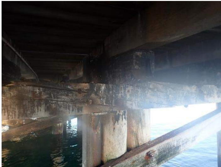
Figure 18 – Typical Condition 6 Timber Crosshead (Defect: Splitting Along Length and Weathering)
