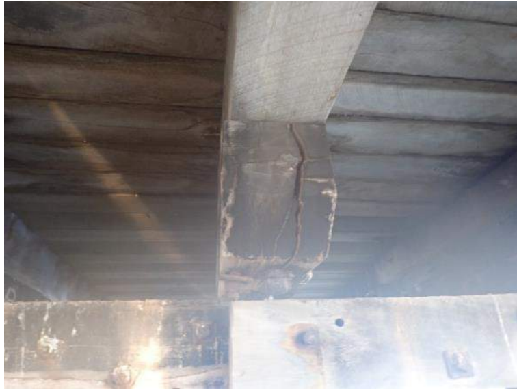
Figure 21 – Typical Condition 5 Timber Corbel (Defect: Weathering & Splitting at End(s) of Member)
