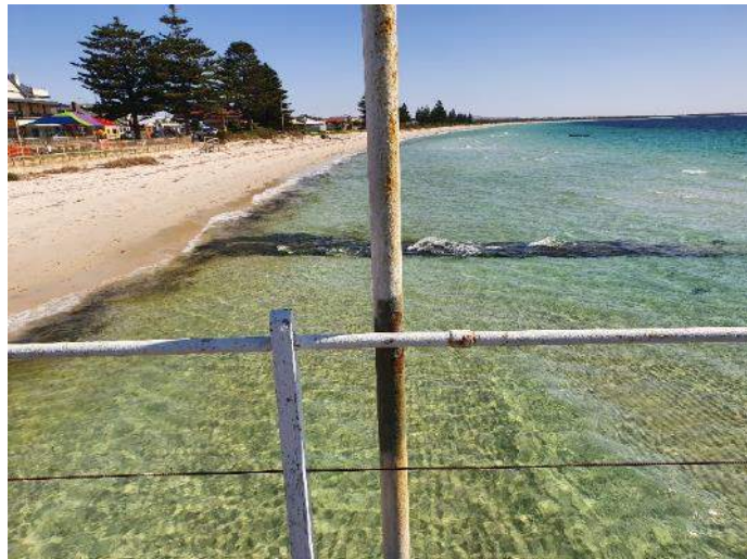
Figure 32 – Typical Condition 4 Light (Defect: Surface Corrosion)
