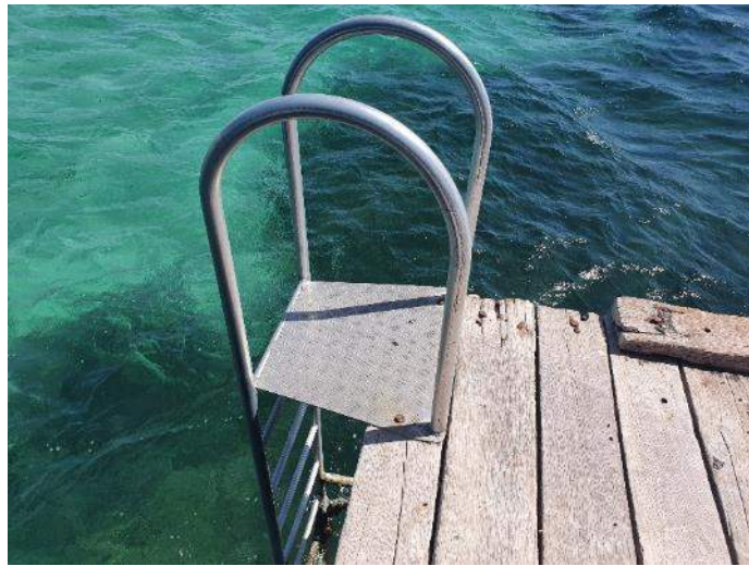
Figure 31 – Typical Condition 3 & 4 Access Ladder (Defect: Corrosion of Fixings)
