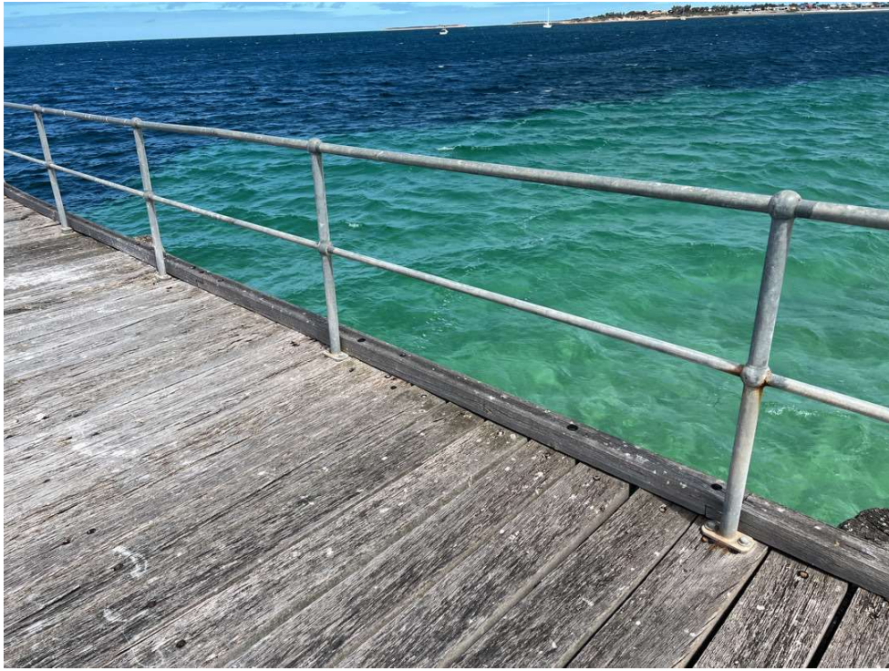
Figure 45: Typical Condition '4' Kerb
