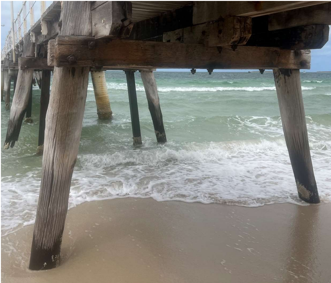
Figure 25: Typical condition '5' Crosshead
