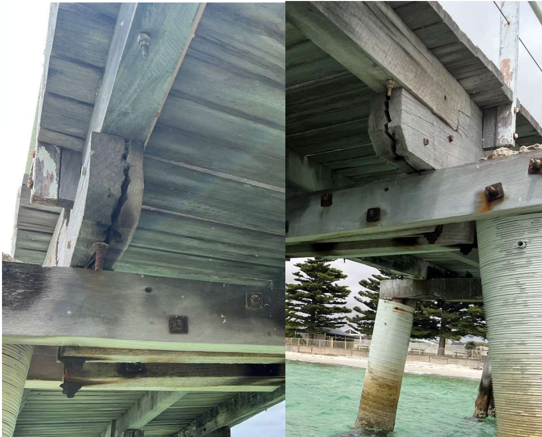
Figure 39 Typical condition '6' Corbel (same corbel-both sides shown)
