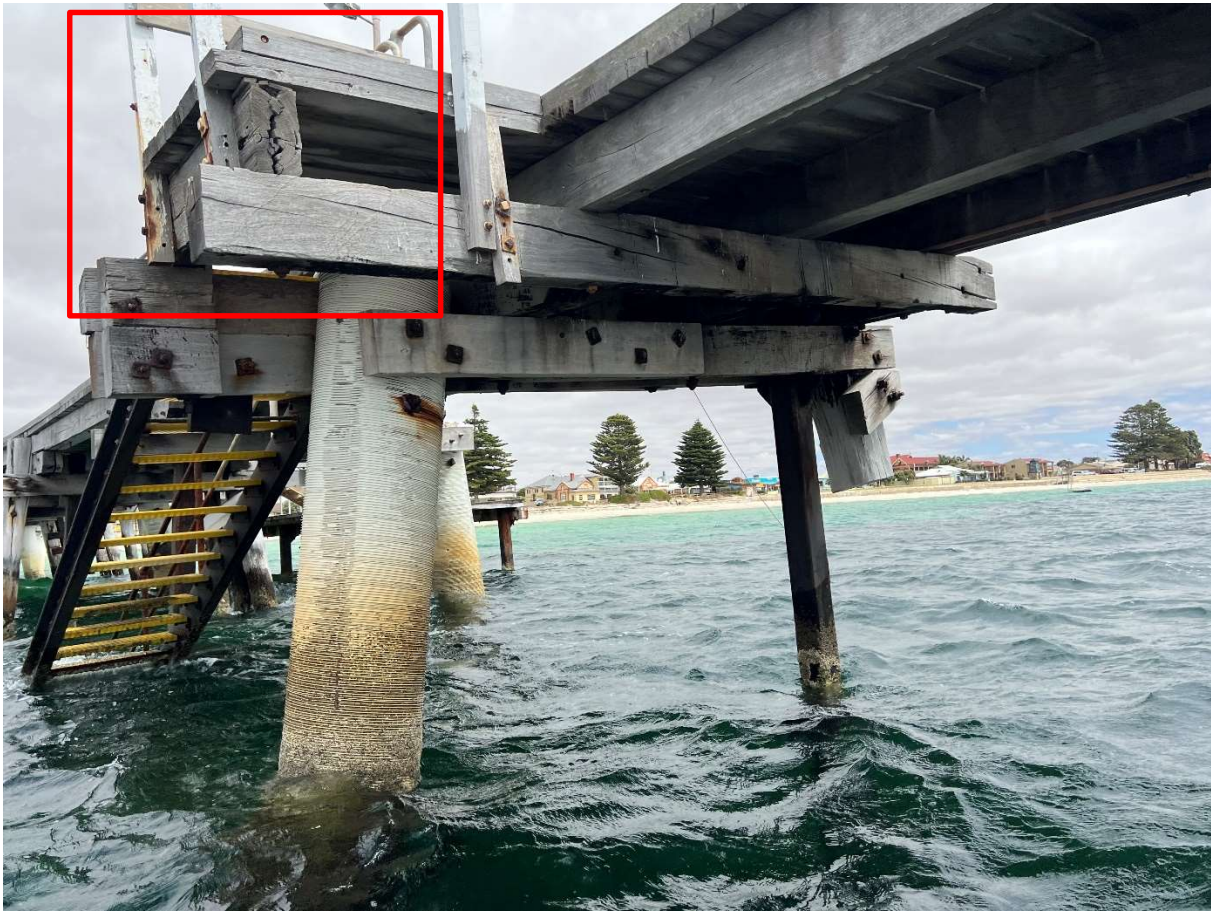
Figure 33 Typical condition '7' girder
