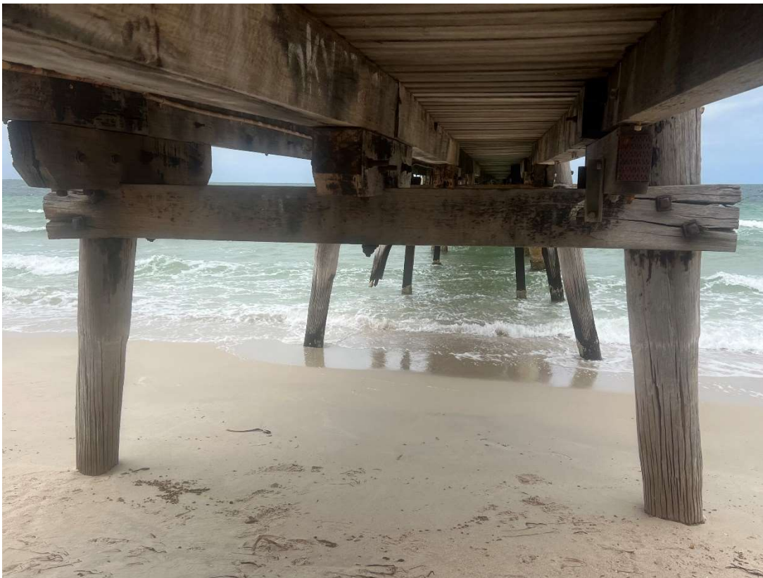
Figure 26: Typical condition '6' Crosshead
