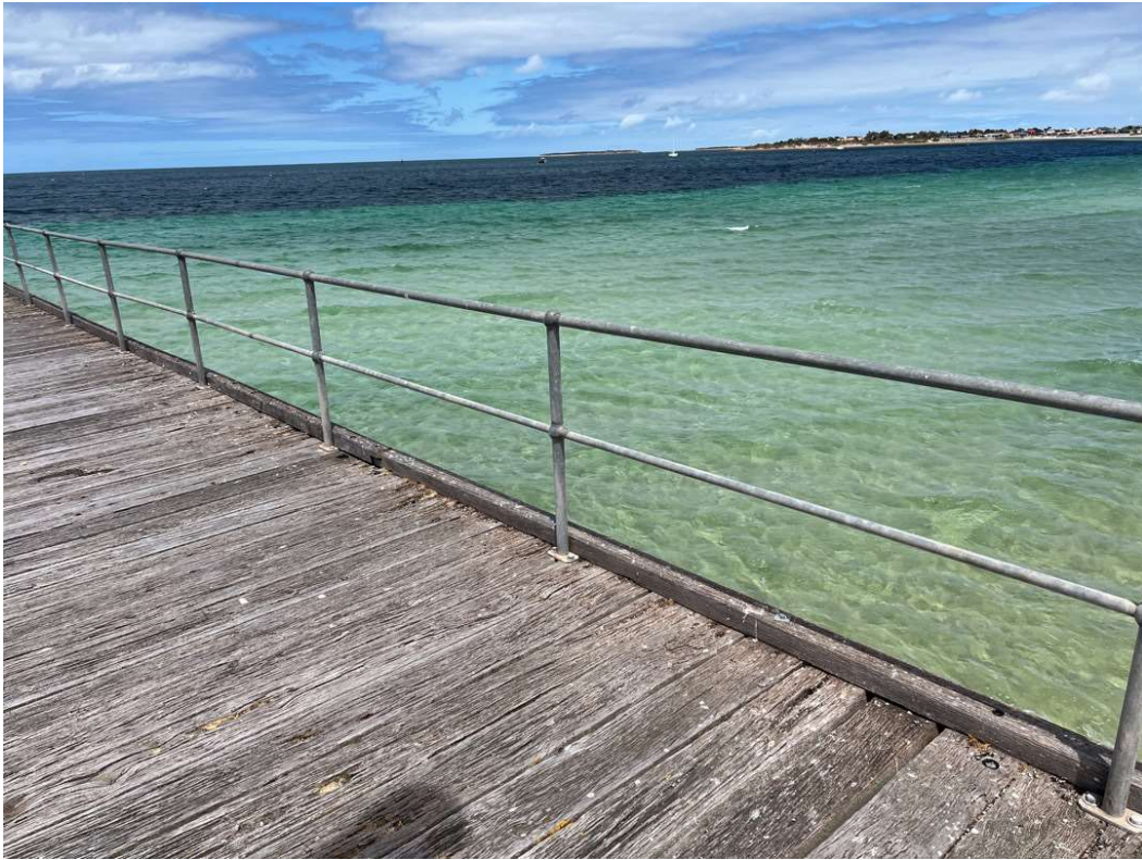
Figure 49: Typical condition '4' of handrail – RHS of the jetty
