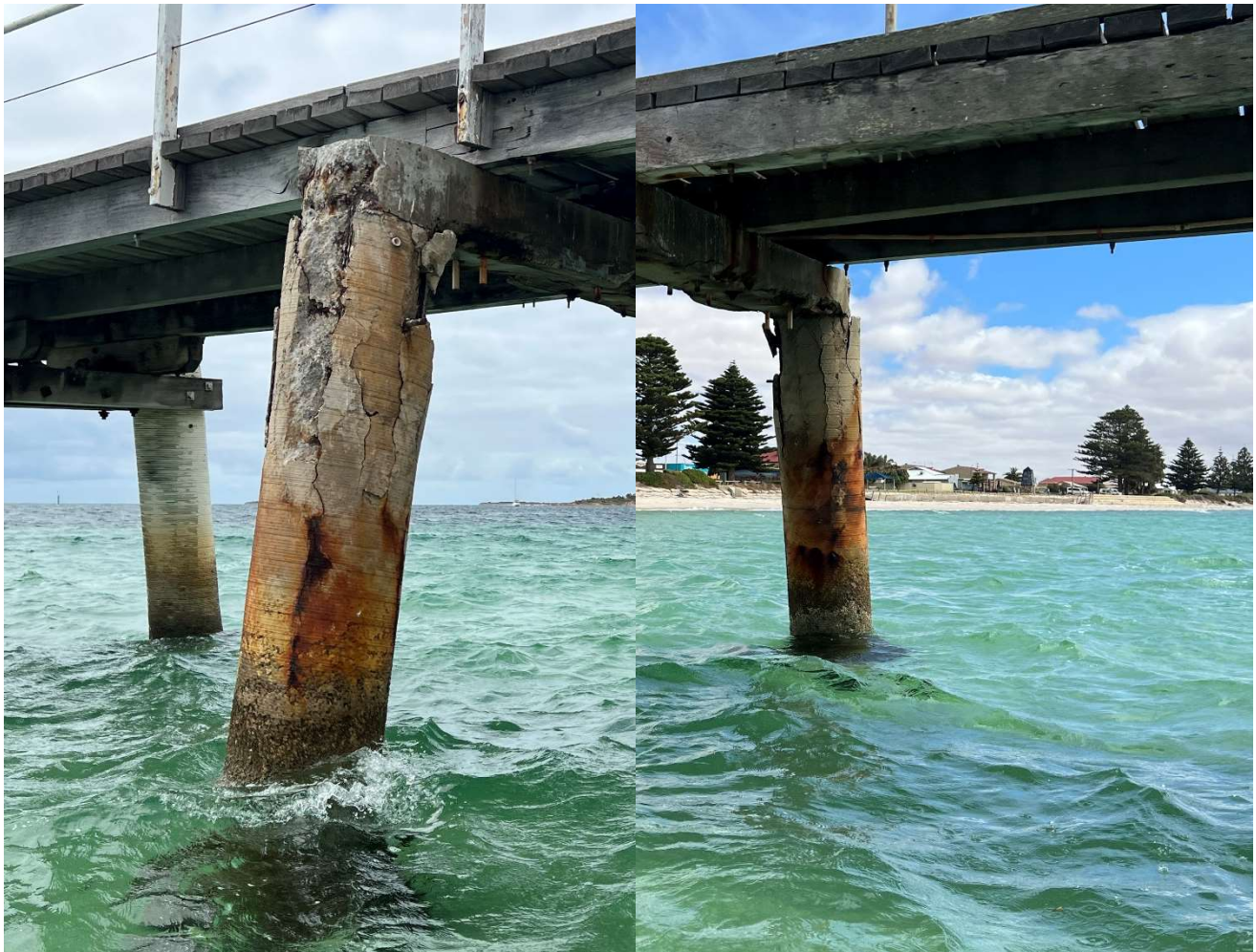
Figure 13: Pile 12A at bent 12, looking from north and south respectively. Condition 6 concrete pile
