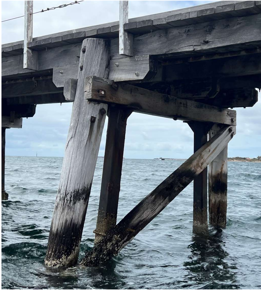
Figure 35 Typical Condition '7' crossbrace. Seaside crossbrace missing
