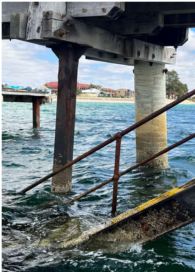
Figure 19 Typical Condition '5' Steel Pile
