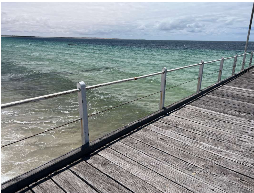
Figure 47: Typical condition '4' of handrail – LHS of the jetty
