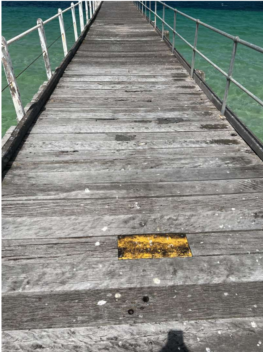
Figure 44 Typical condition '5' decking
