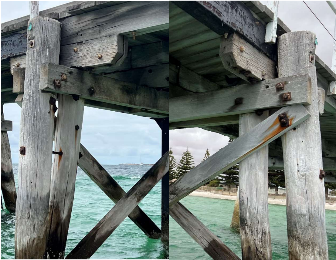
Figure 38 Typical condition '5' Corbel (same corbel-both sides shown)
