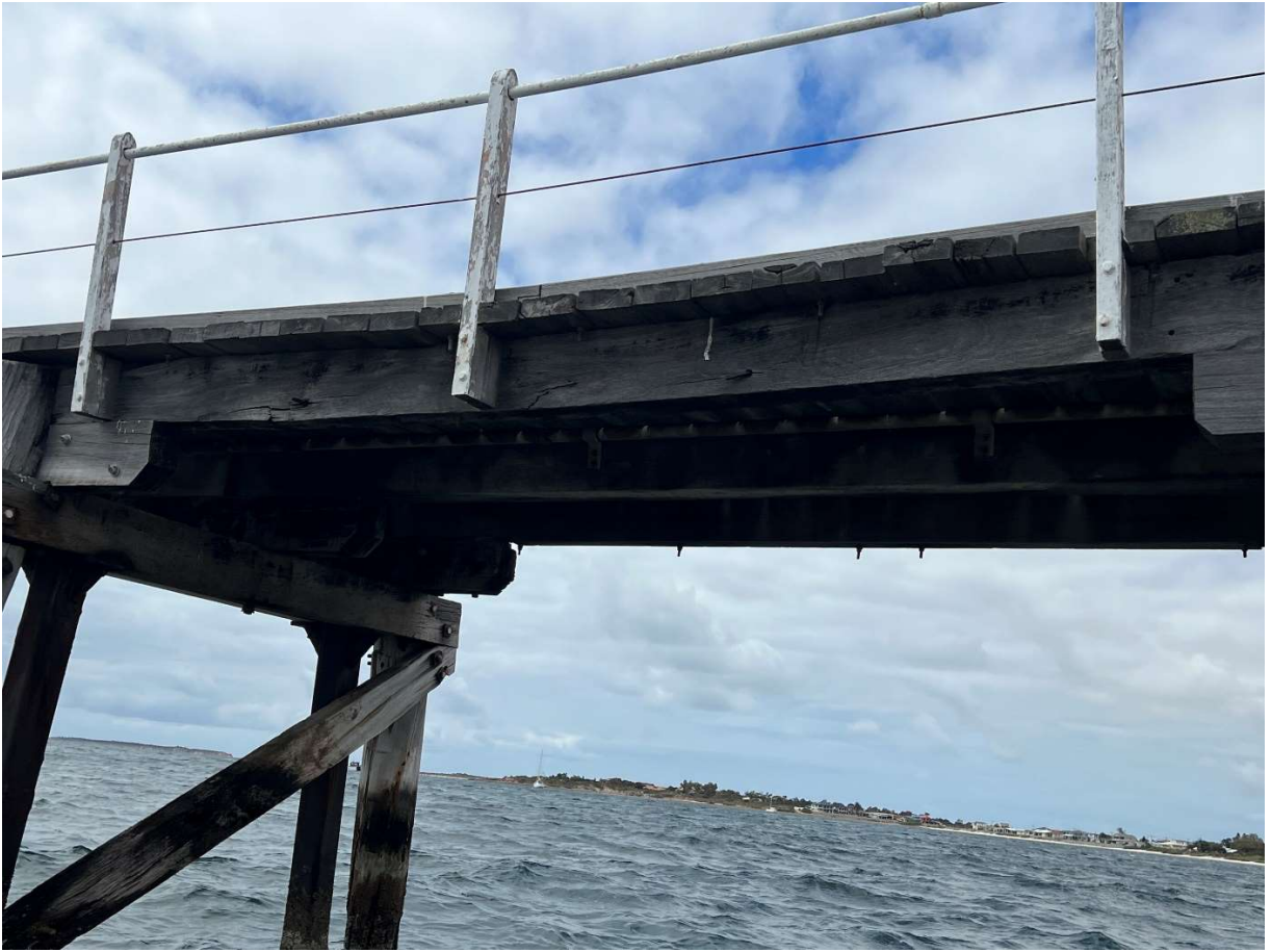
Figure 31: Typical condition '5' girder
