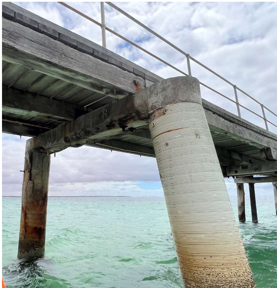
Figure 28 Typical condition '6' concrete crosshead
