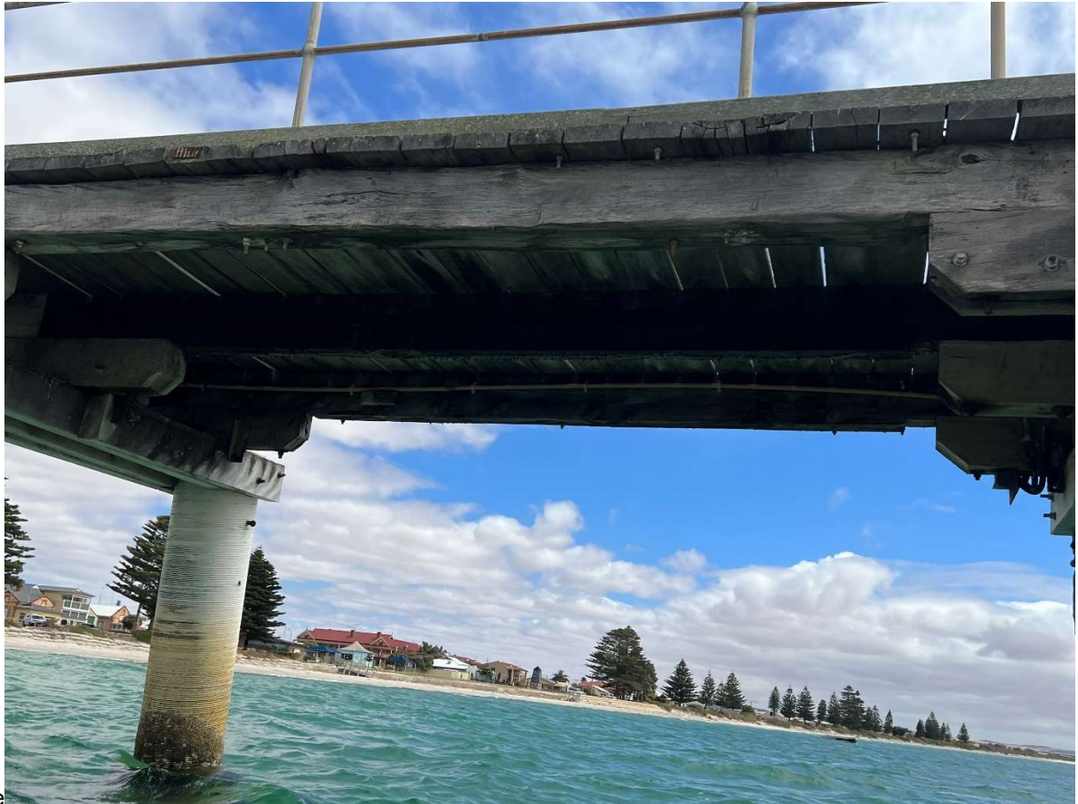
Figure 32 Typical condition '6' girder
