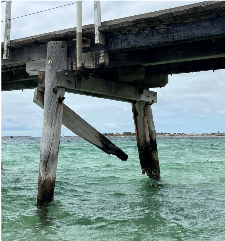
Figure 16: Typical Condition '6' Timber Pile
