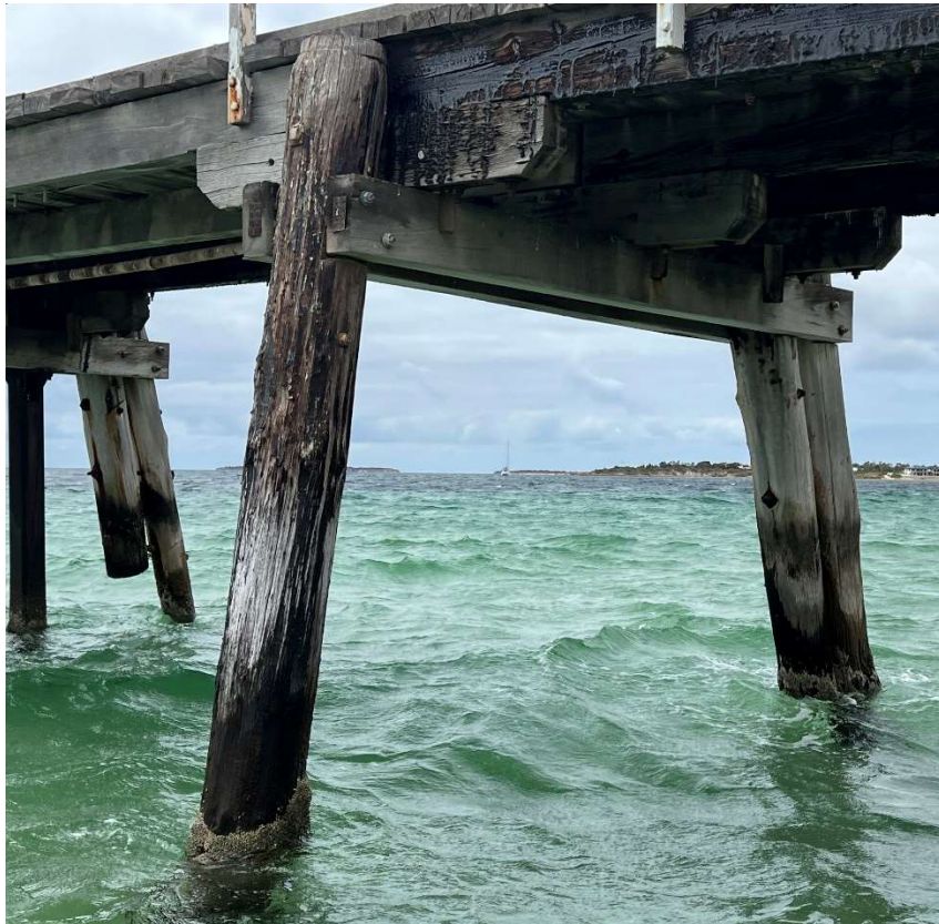
Figure 14: Typical Condition '4' Timber Pile
