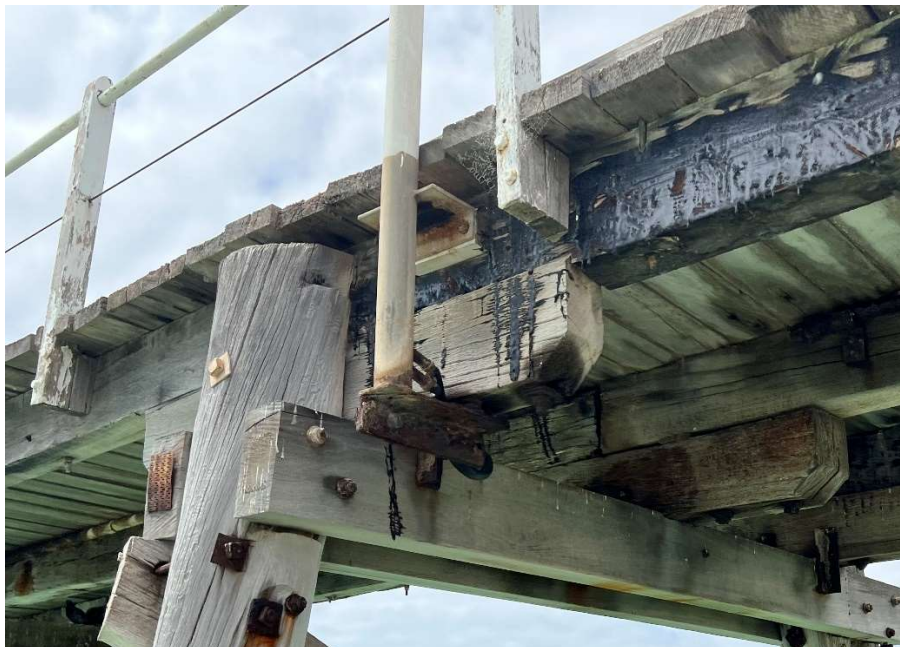
Figure 52 Bent 11 Lightpole corroded connection, rated 6
