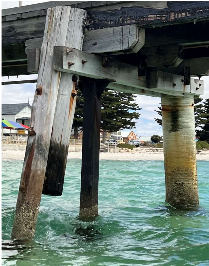
Figure 18 Typical Condition '4' Steel Pile
