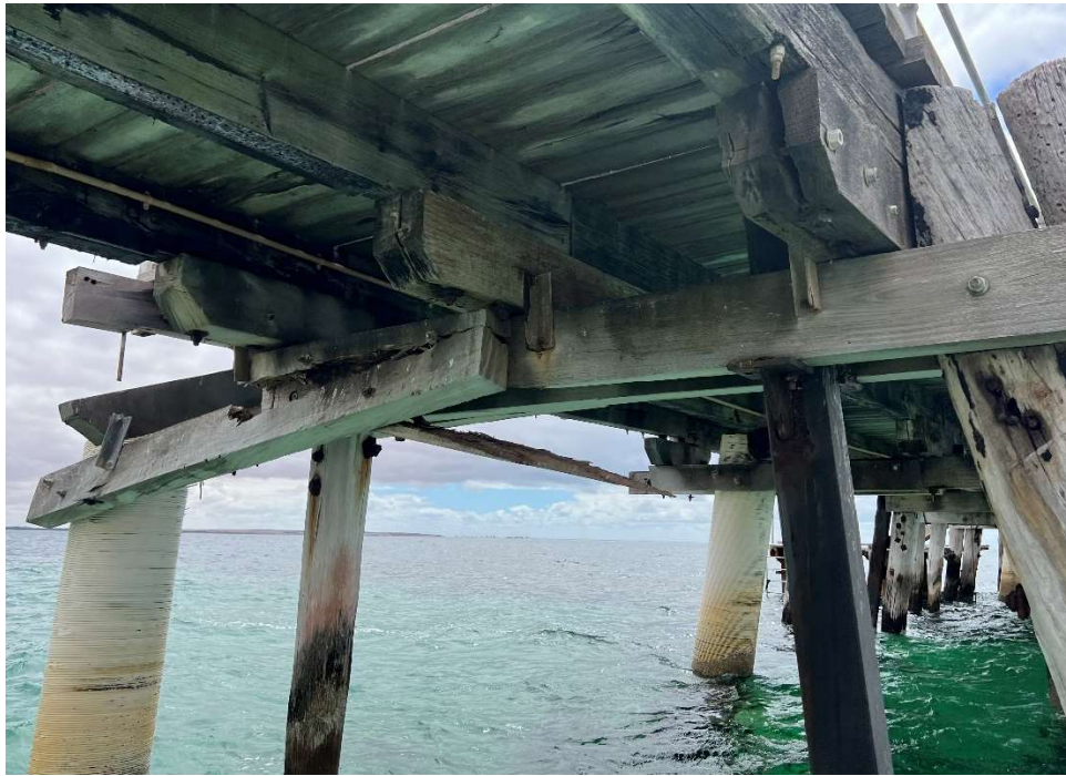
Figure 27 Typical condition '7' Crosshead
