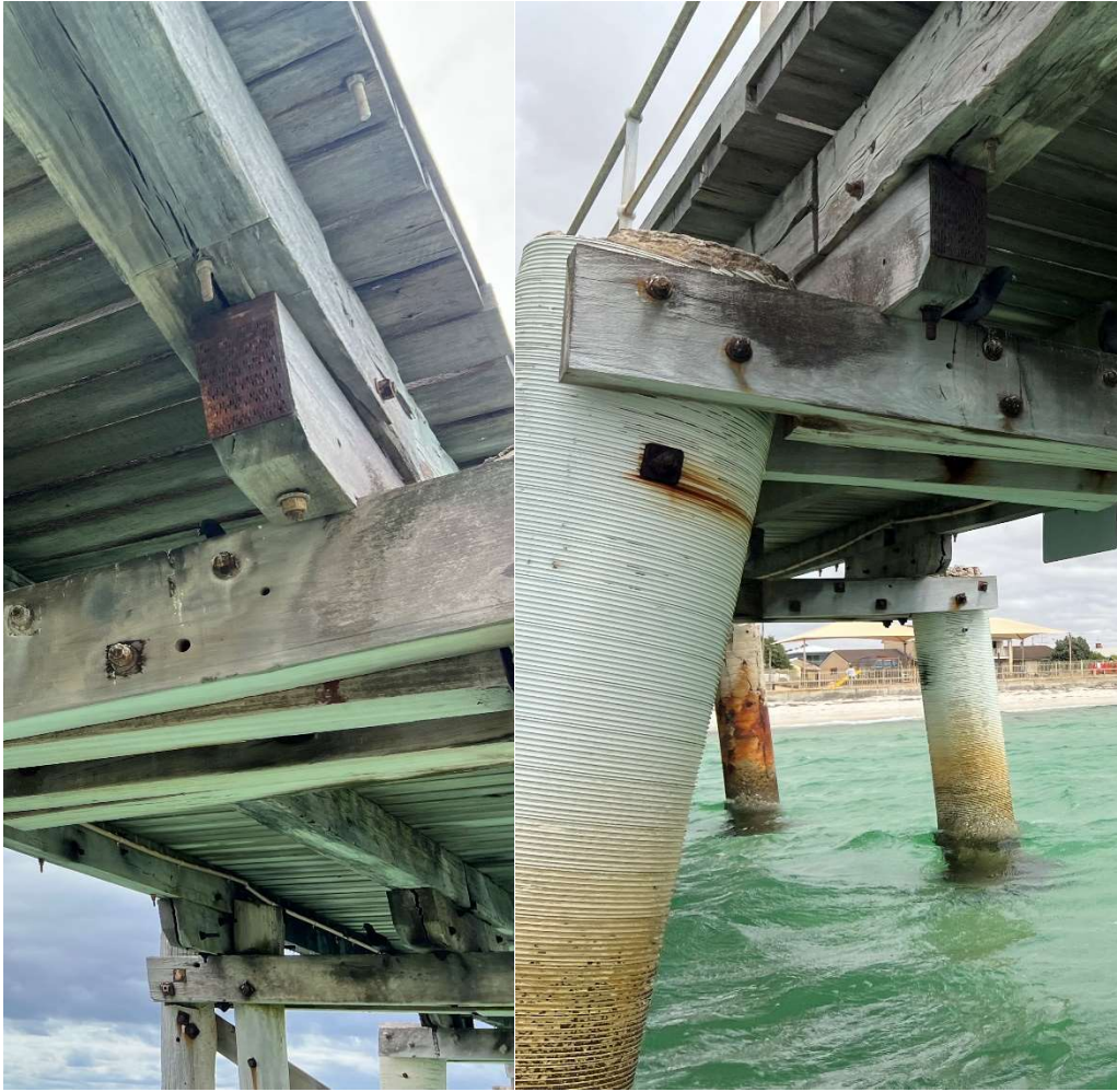
Figure 37 Typical condition '4' Corbel (same corbel-both sides shown)
