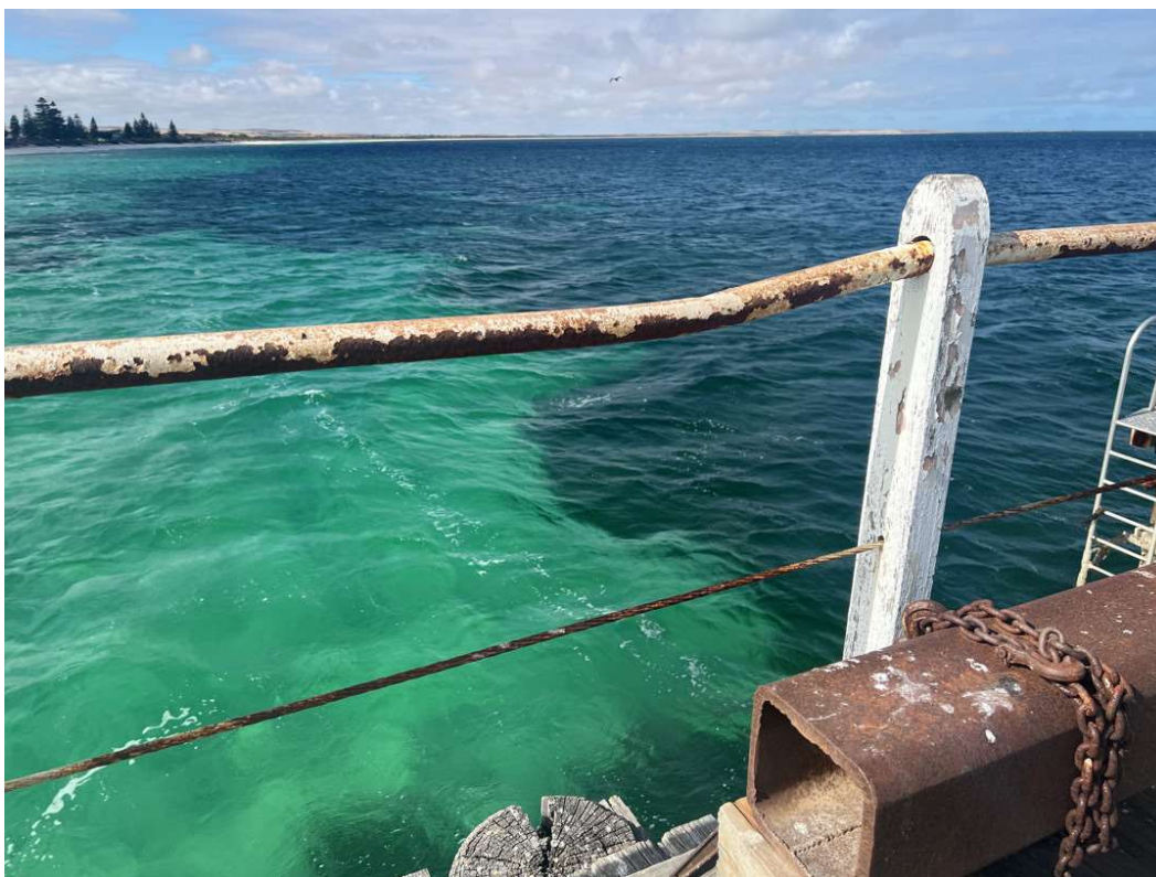
Figure 48 Typical condition '5' of handrail – LHS of the jetty
