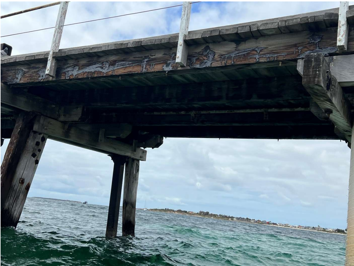
Figure 30: Typical condition '4' girder
