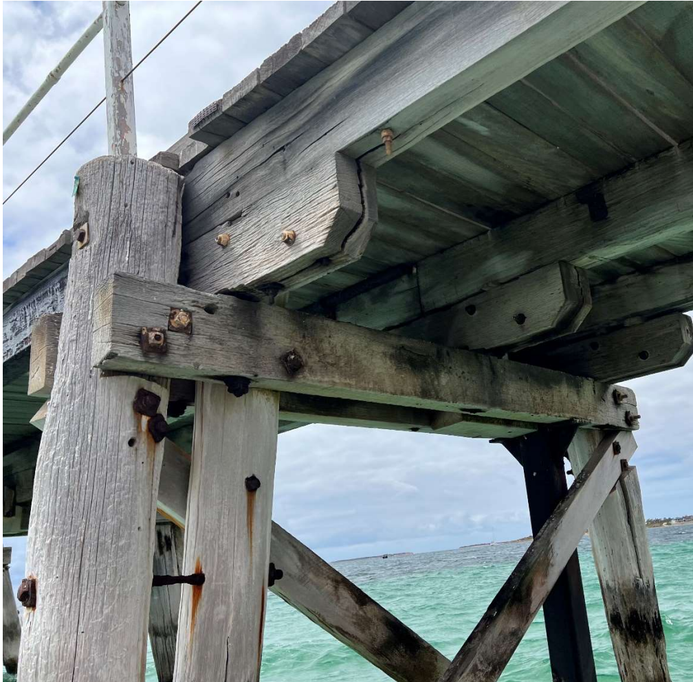
Figure 24: Typical Condition Rating '4' Crosshead
